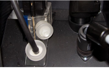
Condensate trap module installed between gas path and O 2 sensor
